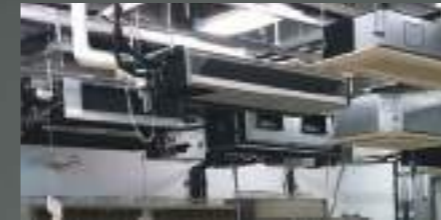
LG Air Conditioning Academy
